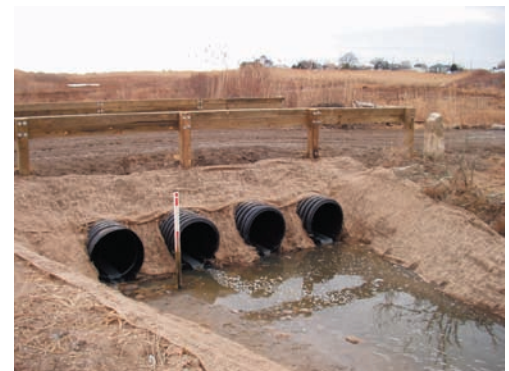
Repairing culverts to restore tidal flow. Photo courtesy of Massachusetts Audubon Society
