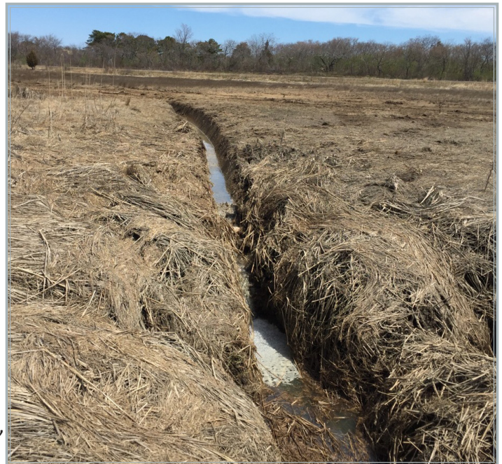
Repairing hydrology of the marsh platform is one of several common approaches to salt marsh restoration. USFWS
