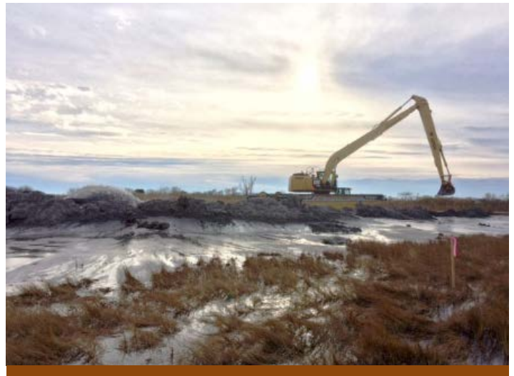
Sediment dredged each year is a valuable resource that could be used in environmentally beneficial ways, such as nourishment of beaches or development of wetland habitats. US Army Corps of Engineers
