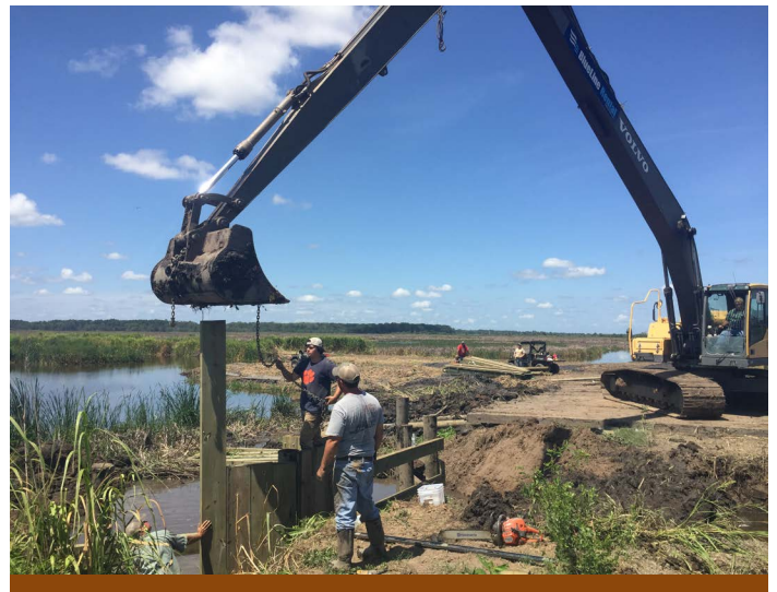
Construction of cross dike and installation of rice trunk to manage water levels for Black Rail. Nemours Wildlife Foundation
